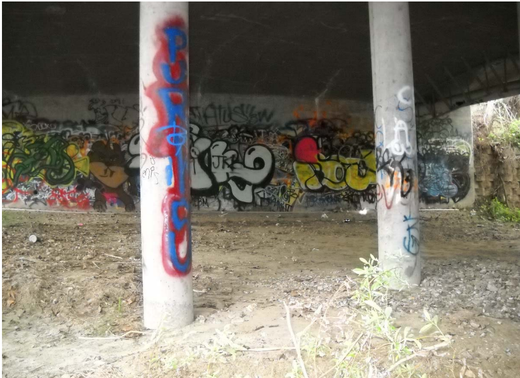
11 FT. DOWNSTREAM OF HEC-RAS RIVER STATION 32+61, LEFT BANK (BENEATH OAK CREEK LN. BRIDGE)
