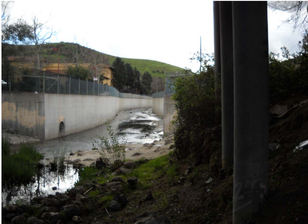
28 FT. DOWNSTREAM OF HEC-RAS RIVER STATION 23+28, DOWNSTREAM DIRECTION (DOWNSTREAM OF REACH NO. 35)
